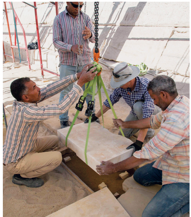
Pavement laying by Saber, Mohamed, Johannes, and Tayib, January 2019. Photo: Frank Helmholz.
