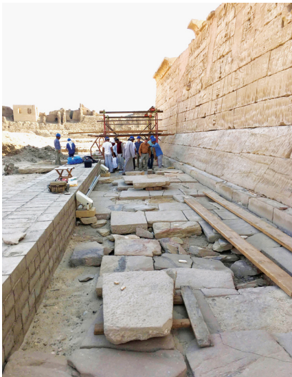
Western pavement before restoration, November 14, 2018. Photo: Ray Johnson.
